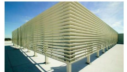
5. PENTHOUSE EQUIPMENT - SCREEN
