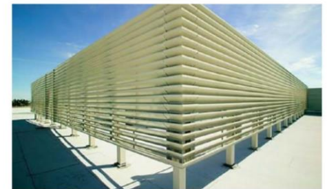
5. PENTHOUSE EQUIPMENT - SCREEN
