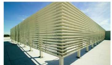
5. PENTHOUSE EQUIPMENT - SCREEN
